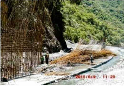
(c) 擋土牆牆身鋼筋遭土石覆蓋災損
